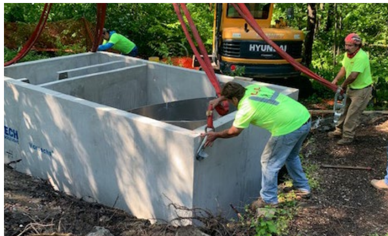
Installation of the filtration system as part of Awbury's pond and watercourse restoration project. Photo Credit - Branda O'Neil
